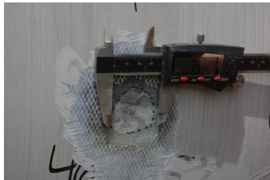
(b) Removal of Some Glass Layers
