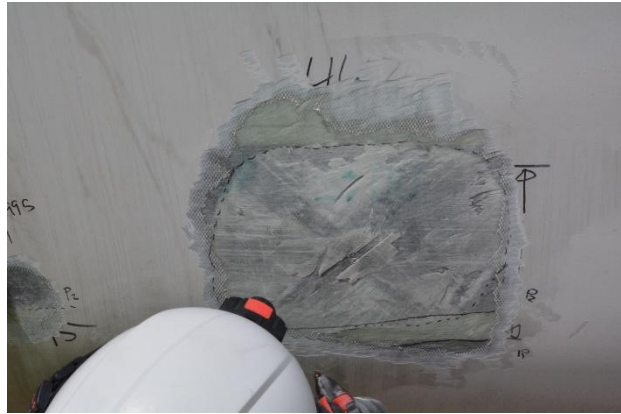
(b) Removal of Some Glass Layers
