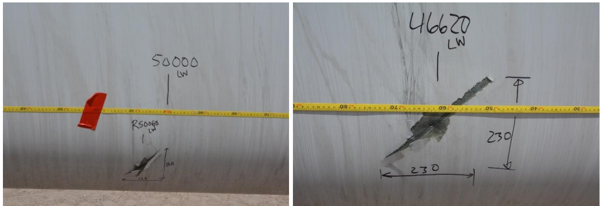
Figure 12: Examples of Lightning Strike Damage Annotated During Initial Inspection
