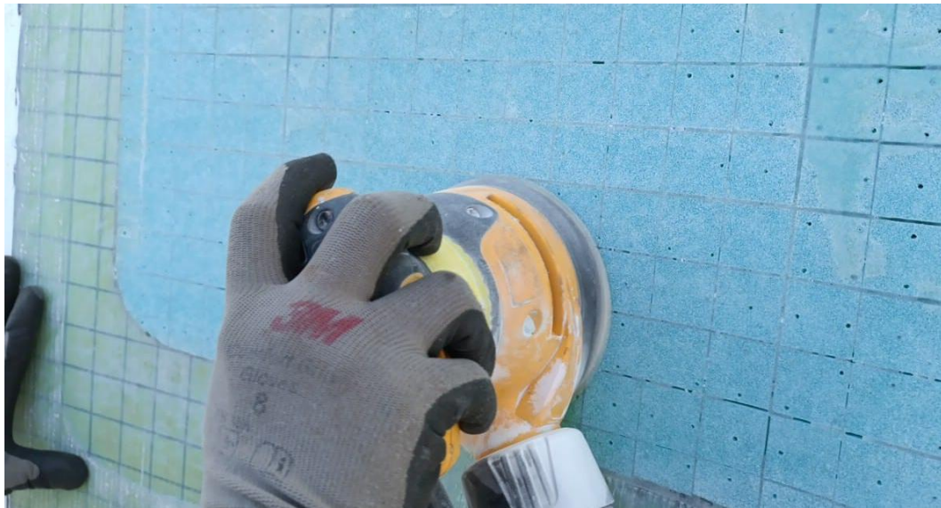
Figure 25: Example of the Final Sanding of a Glass Repair over Foam Core
