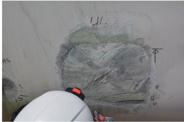
(b) Removal of Some Glass Layers
