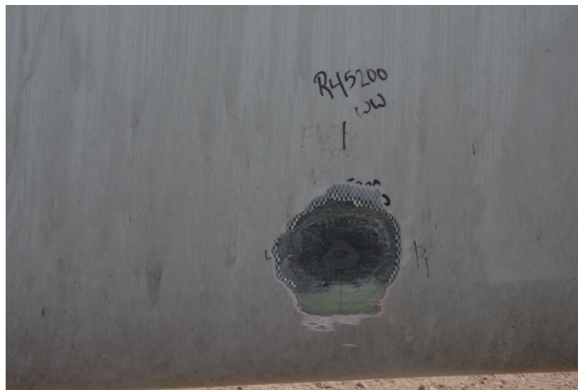
Figure 15: Illustration of a Grind to the Bottom of a Lightning Damage to a Carbon Spar Cap
