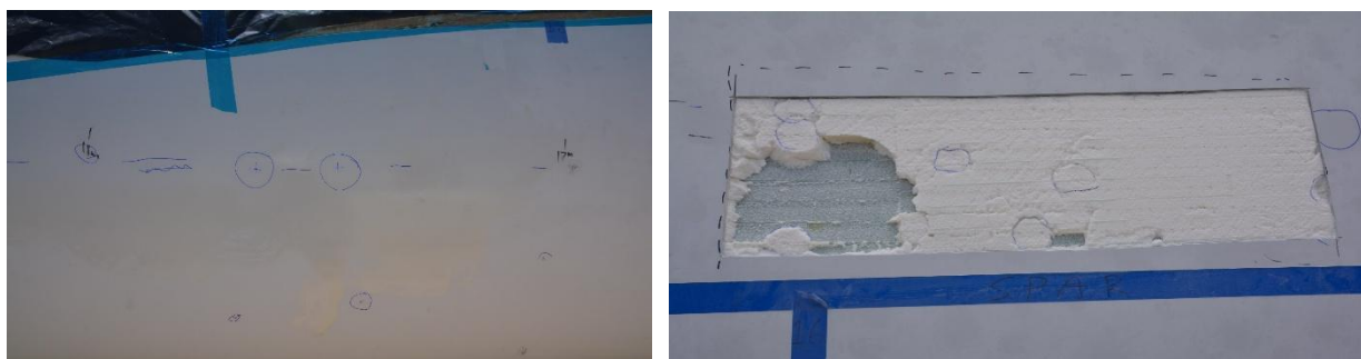
(a) Small Exterior Indications (b) Internal Damage Revealed by Destructive Inspection
