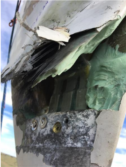
(a) Significant Delamination
