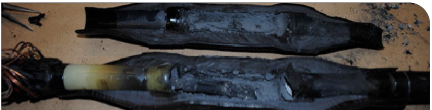
Figure 5 Example of a dissected compression coupling showing extreme heat, burning, and charring. Subsequent dissection of the actual coupling showed no sign of wire brushing (Photograph courtesy of Imcorp).
