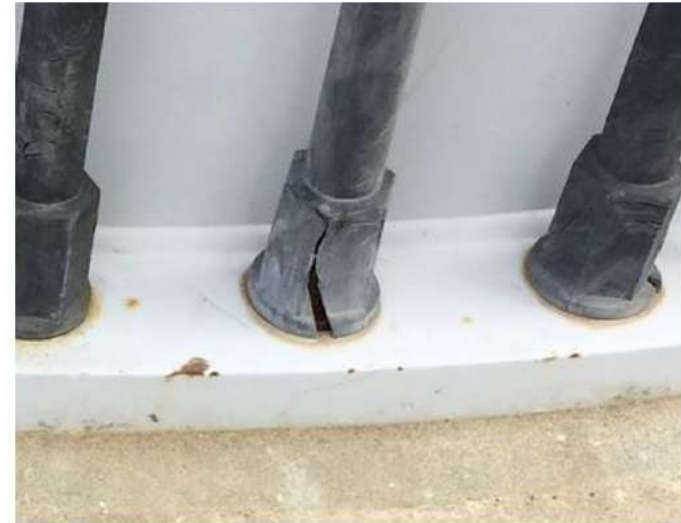
Anchor bolt cover failure
