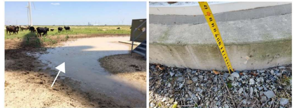
Figure 14. Poor grading resulting in pooling of water in left photo and example of low backfill height in right photo.
