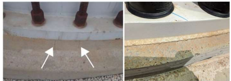
Figure 10. Radial cracking in cementitious grout in left photo and circumferential cracking in epoxy grout shown in right photo.
