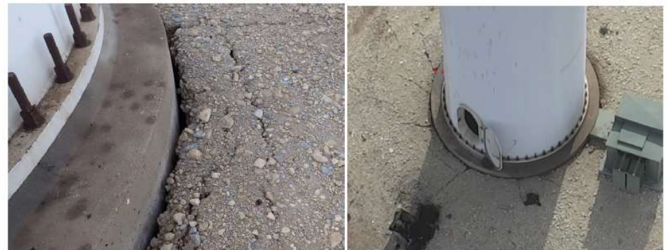
Figure 18. Gap between pedestal and backfill from close-up in left photo and aerial view of foundation soil cracking in right photo.
