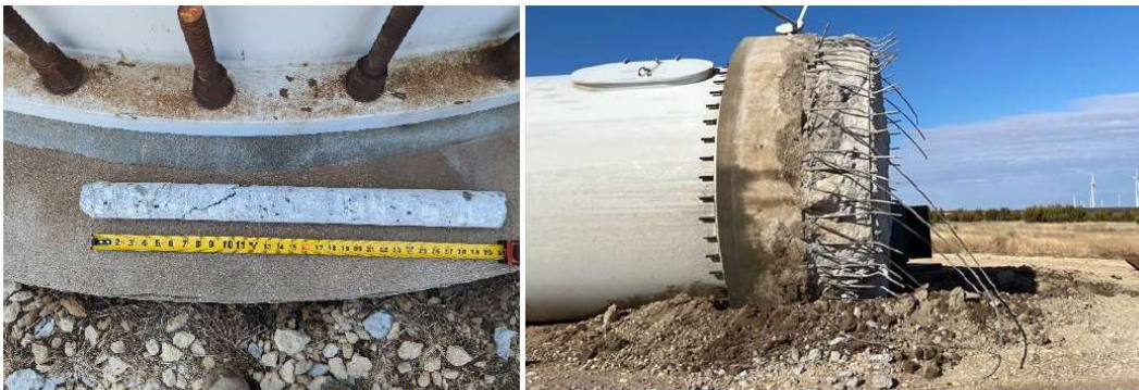
Figure 2019. Cracked concrete core taken at the anchorage pullout area in the left photo, turbine collapse due to foundation overloading event and anchorage pullout failure in the right photo.
