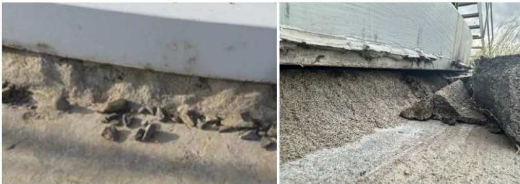
Figure 13. Loss of grout with the potential for gapping shown in the left photo and significant loss of grout with gapping due to low anchor bolt tension shown in right photo.
