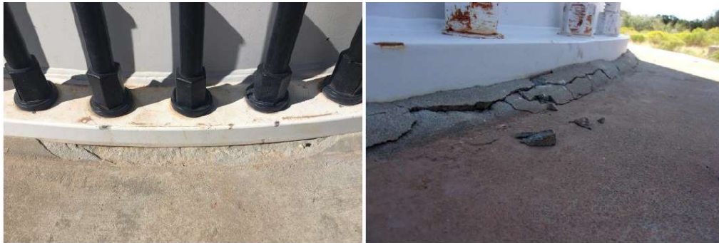
Figure 9. Early-stage spalling in left photo and late-stage spalling with significant cracking in right photo.
