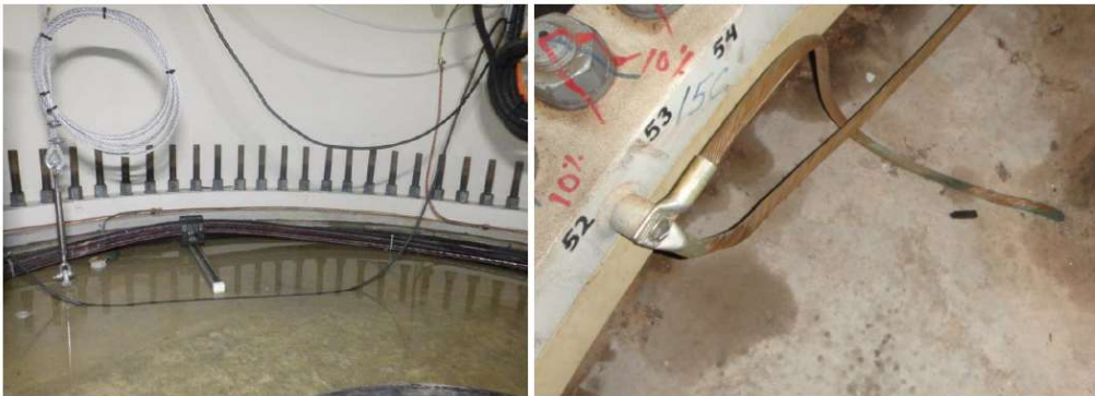
Figure 15. Water pooled shown in left photo and corrosion of grounding cables due to water in the basement shown in left photo.
