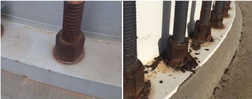
Figure 16. Hardware with surface corrosion is shown in the left photo and hardware with advanced corrosion is shown in the right photo.
