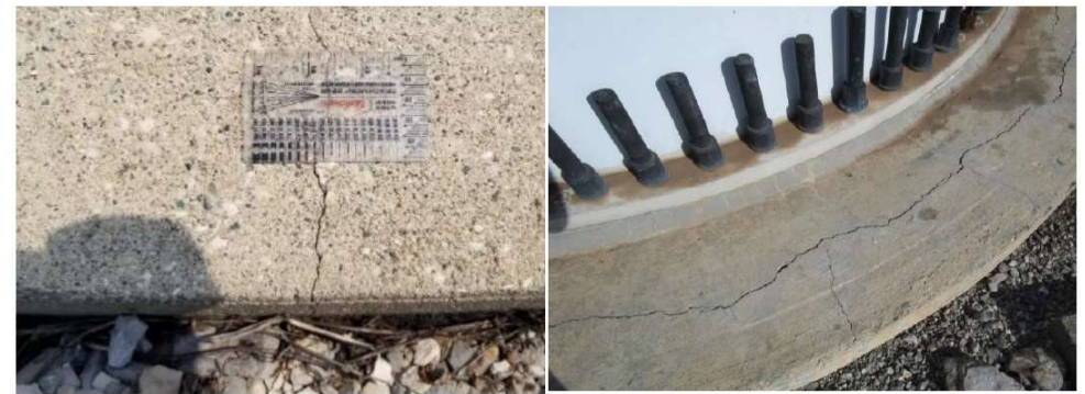
Figure 12. Pedestal radial shrinkage crack in left photo and more significant circumferential cracking in the right photo.
