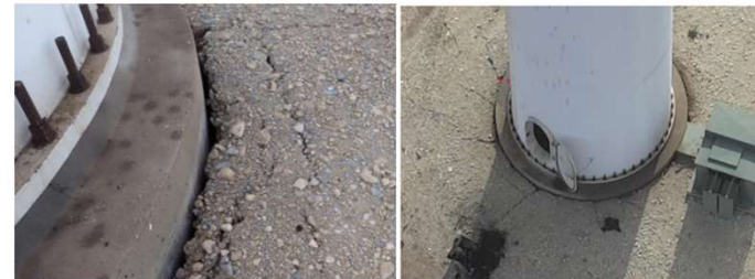
Figure 18. Gap between pedestal and backfill from close-up in left photo and aerial view of foundation soil cracking in right photo.
