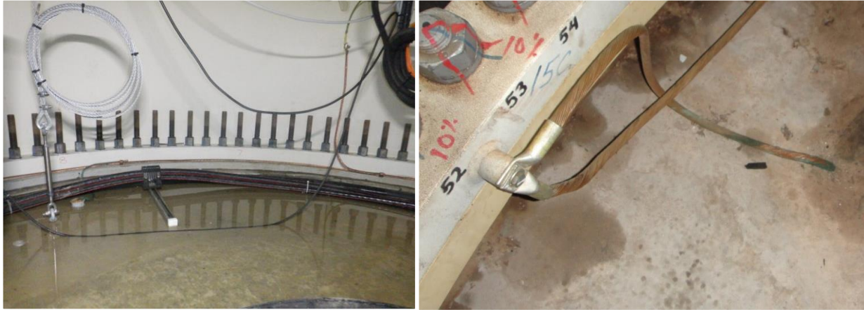
Figure 15. Water pooled shown in left photo and corrosion of grounding cables due to water in the basement shown in left photo.
