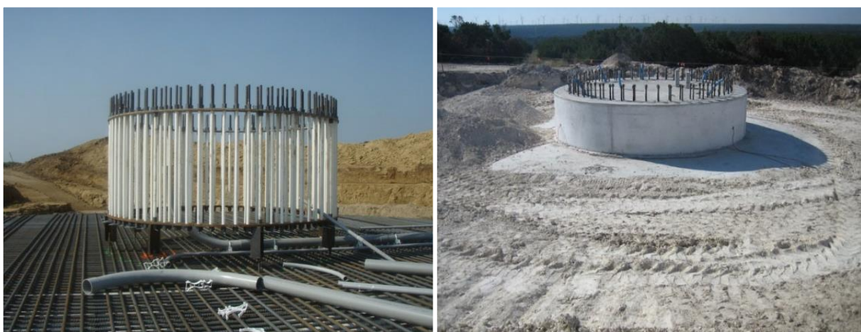
Figure 7. Anchor bolt/embedment plate assembly prior to concrete placement shown in left photo and fully constructed foundation in the right photo.
