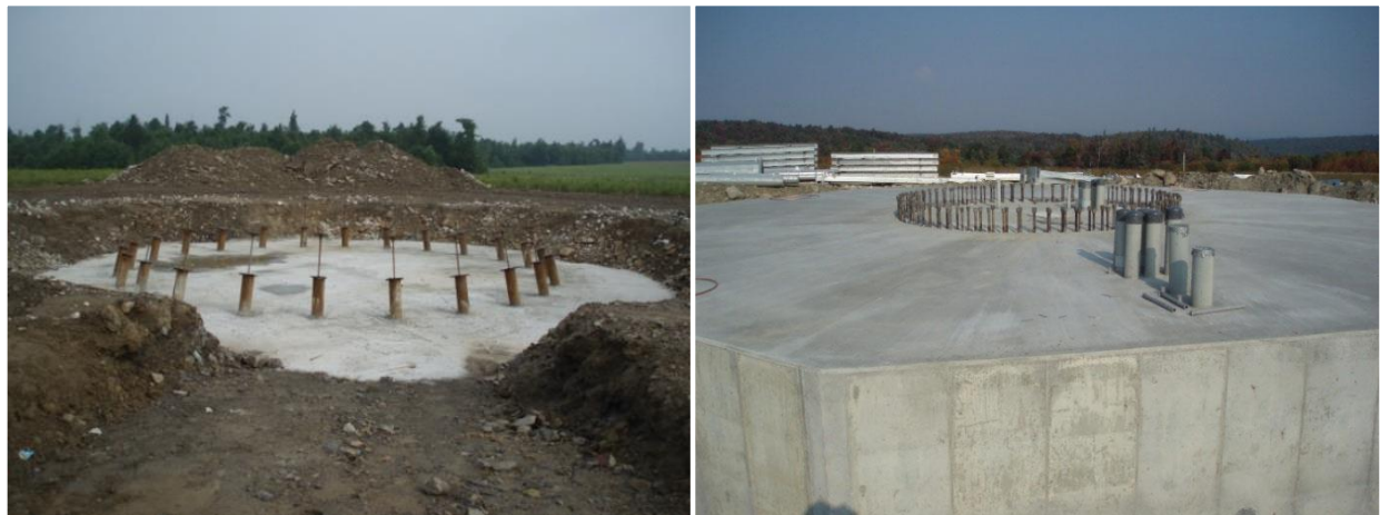
Figure 5. Pile supported cap foundation in construction in left photo and completed foundation in right photo.
