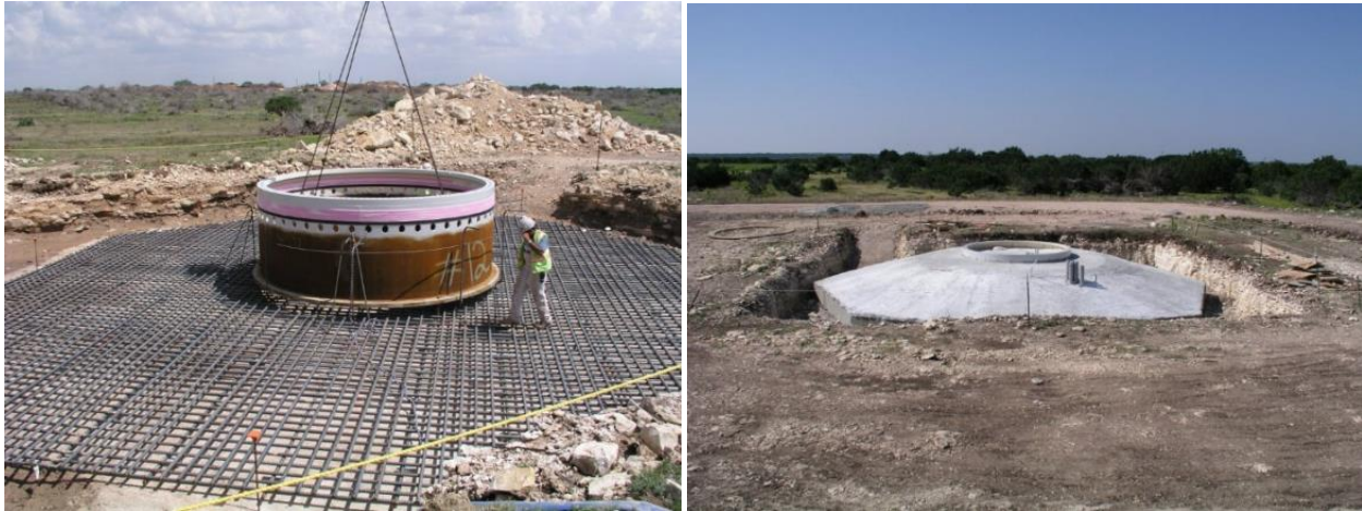
Figure 8. FMP connection prior to construction of foundation in left photo and fully constructed FMP style foundation prior to backfill shown in right photo.
