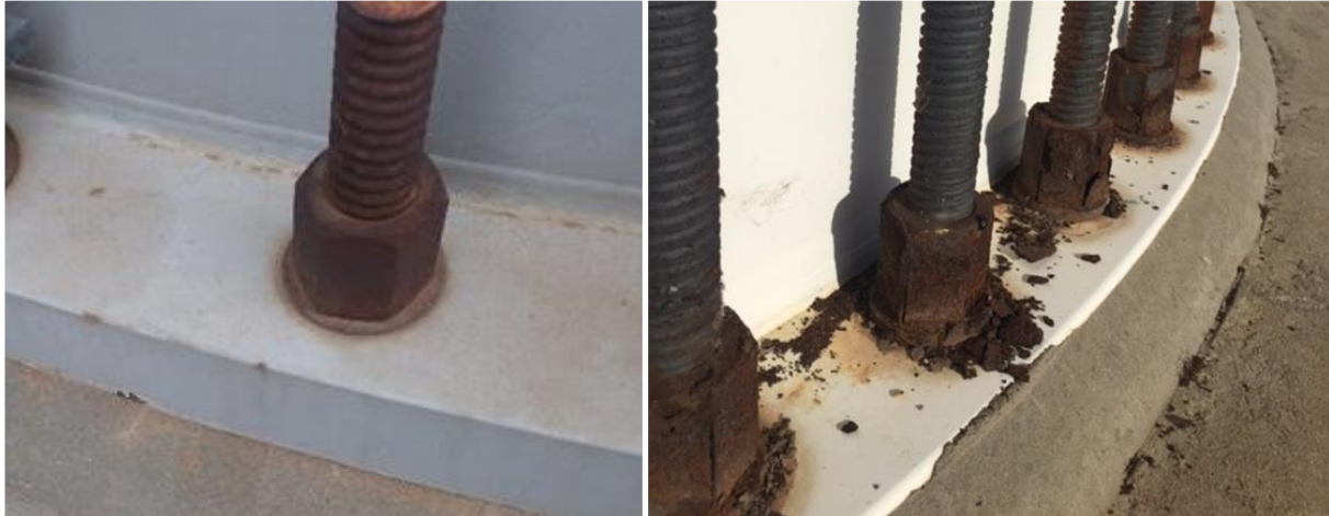
Figure 16. Hardware with surface corrosion is shown in the left photo and hardware with advanced corrosion is shown in the right photo.
