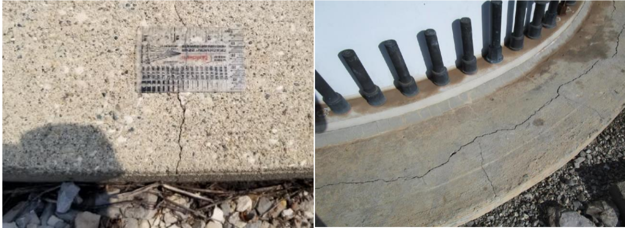
Figure 12. Pedestal radial shrinkage crack in left photo and more significant circumferential cracking in the right photo.
