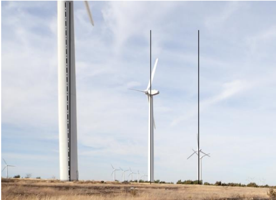
Figure 21. Example of a foundation out of level resulting in visually observable tower tilt compared to neighboring turbines. Solid vertical lines are drawn representing two plumb and vertical towers to the right whereas the tower on the left has a tower centerline, shown with a dashed line, that is not plumb.
