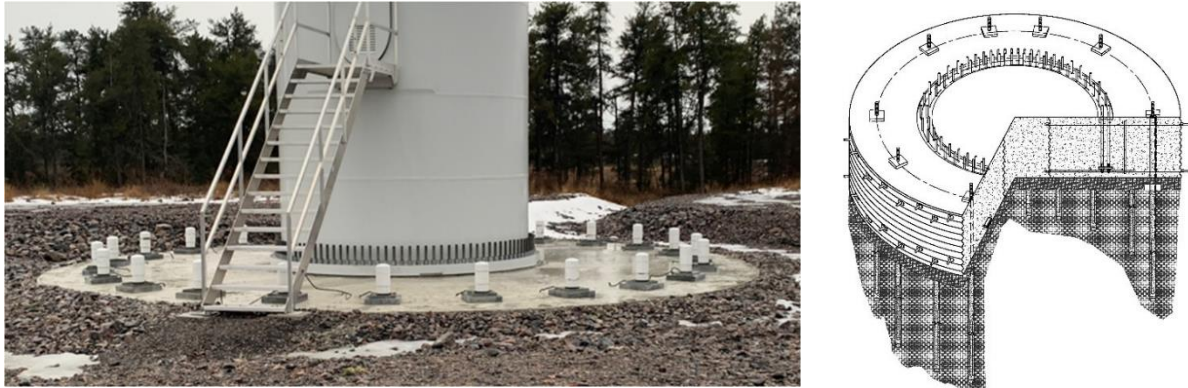
Figure 4. Rock anchor foundation in service in left photo, and three-dimensional image illustrating the design elements of the rock anchor foundation in the right photo.
