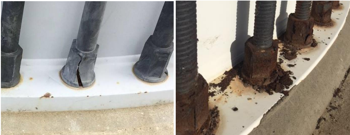
Figure 17. Cracked bolt cover shown in the left photo and a bolt and nut with the cover removed wherein water was being trapped resulting in corrosion of the lower portion of the nut is shown in the right photo.
