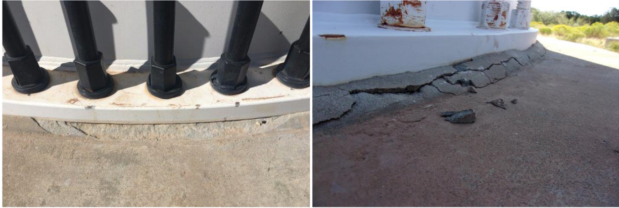
Figure 9. Early-stage spalling in left photo and late-stage spalling with significant cracking in right photo.
