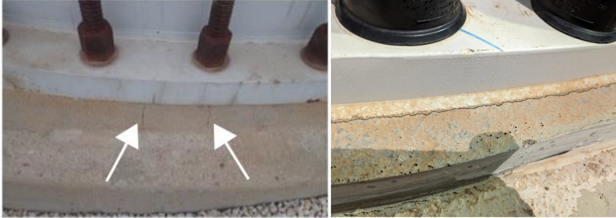
Figure 10. Radial cracking in cementitious grout in left photo and circumferential cracking in epoxy grout shown in right photo.
