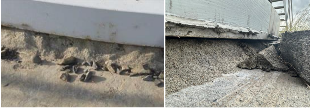
Figure 13. Loss of grout with the potential for gapping shown in the left photo and significant loss of grout with gapping due to low anchor bolt tension shown in right photo.
