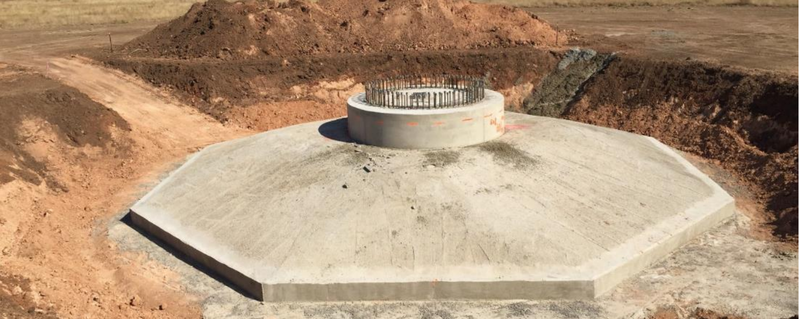
Figure 2. Typical gravity-based spread footing foundation in construction state prior to being covered with backfill.
