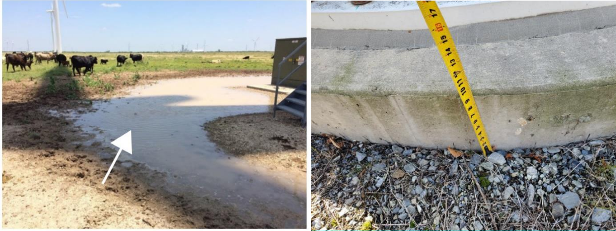
Figure 14. Poor grading resulting in pooling of water in left photo and example of low backfill height in right photo.
