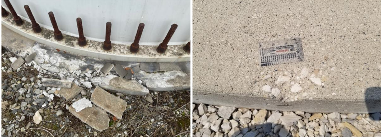
Figure 11. Structurally significant pedestal spalling in left photo and minor debris/impact pedestal spalling in right photo.
