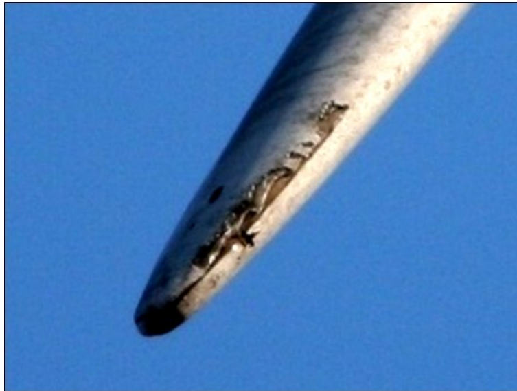
Figure B: Example of Blade Damage Documented with Ground-based Digital Photography.
