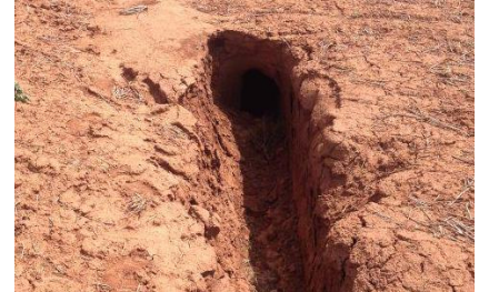
Figure 6 Improper compaction allows for water infiltration, erosion, and eventual lack of heat conduction potentially causing cables to overheat and fail prematurely
