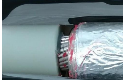
Figure 5 Improper accessory alignment. Was in service for 1.25 years before detection (image courtesy of IMCORP)
