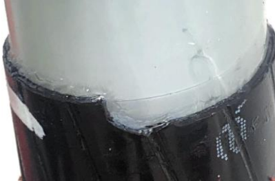
Figure 4 Improper insulation screen cutback and insulation score due to improper tool setup (image courtesy of IMCORP)
