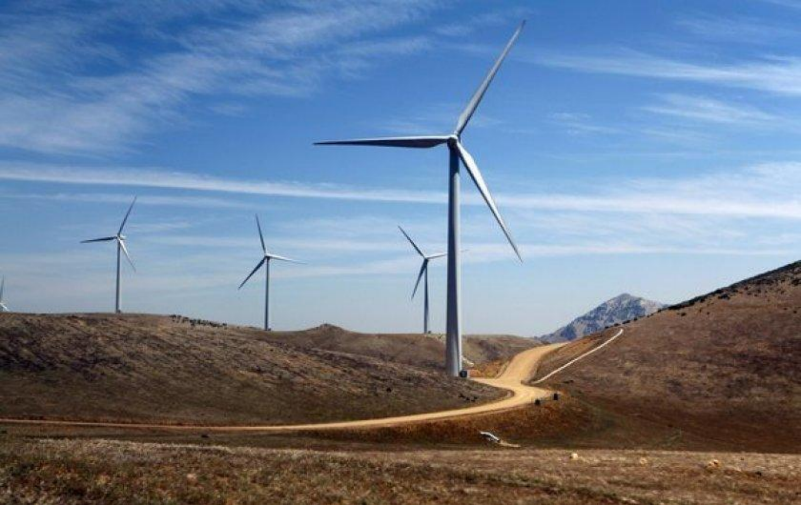
Wind turbines are seen at the Los Angeles Department of Water and Power's Pine Tree Wind Farm in the Tehachapi Mountains. (Los Angeles Times)
