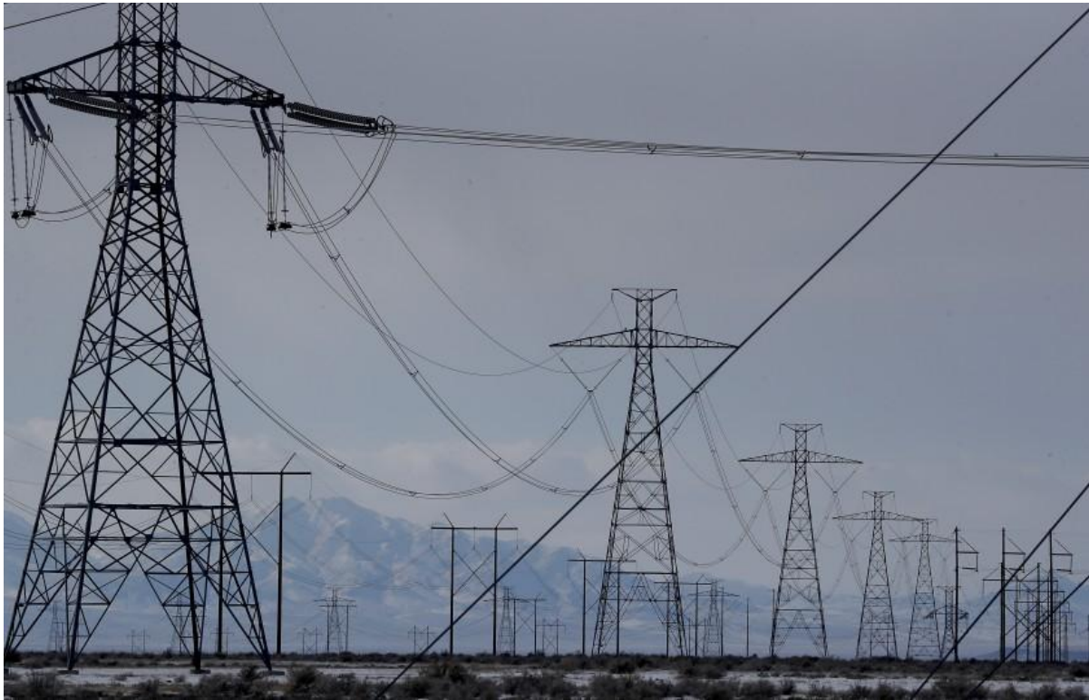
Power from the coal-fired Intermountain Power Plant in Delta, Utah, travels 488 miles to Adelanto, Calif., and then to L.A. (Luis Sinco / Los Angeles Times)
